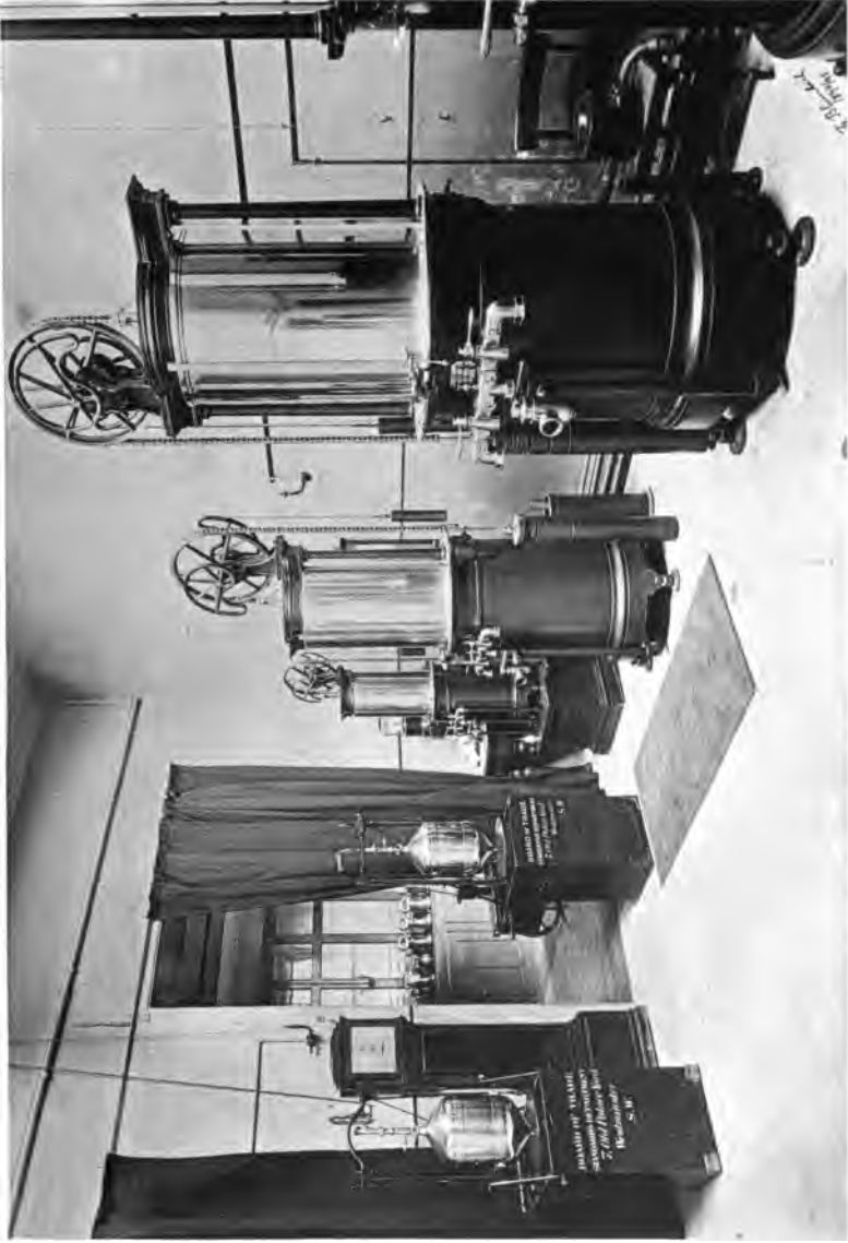
Fig. 16.—GAS-ROOM, STANDARDS OFFICE. Showing the 10, 5, and 1 cubic foot Standards.
